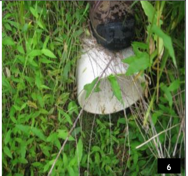
Under drain pipe collects runoff from the bottom of the rain garden and discharges it down-gradient (which may be a good option if you have poor infiltration rates)
