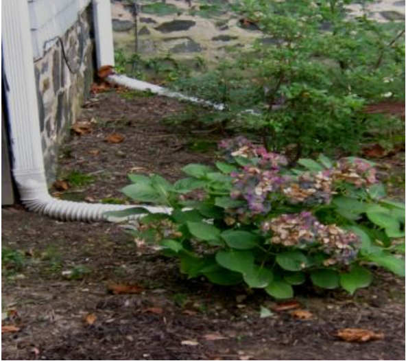
Two downspouts, one rain garden and a large area of conservation landscaping
